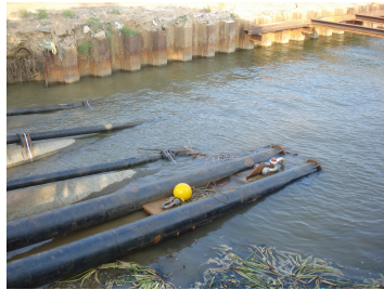
Figure 23: Landfill point: Pipes entering the water 1
