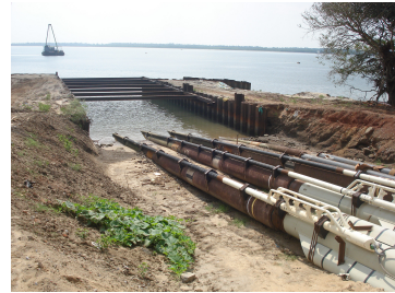
Figure 24: Landfill point: Pipes entering the water 2
